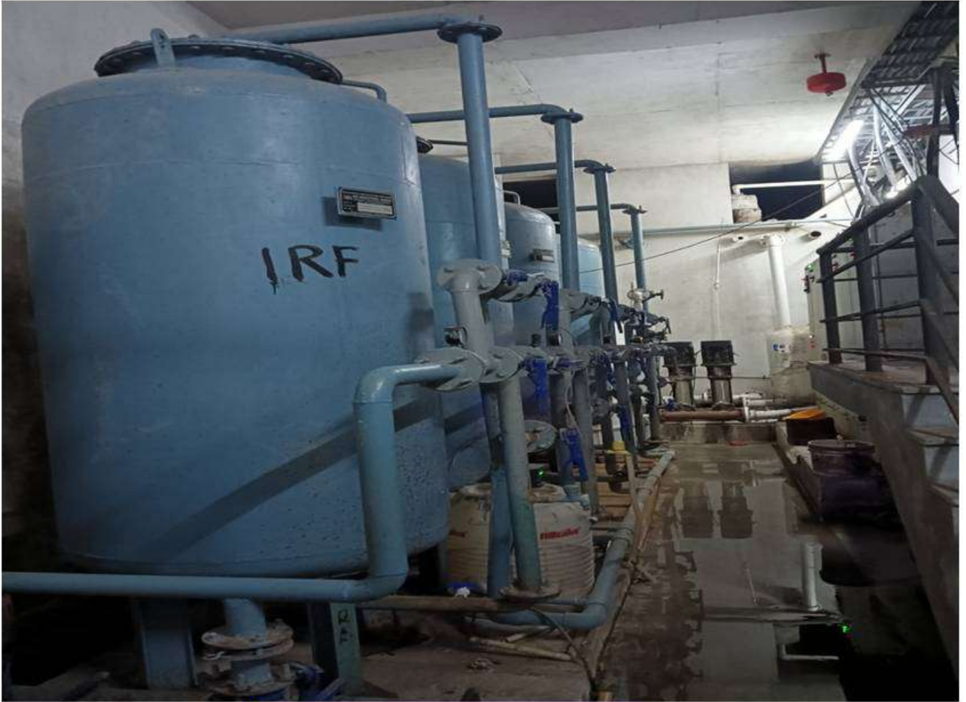
Water treatment plat
