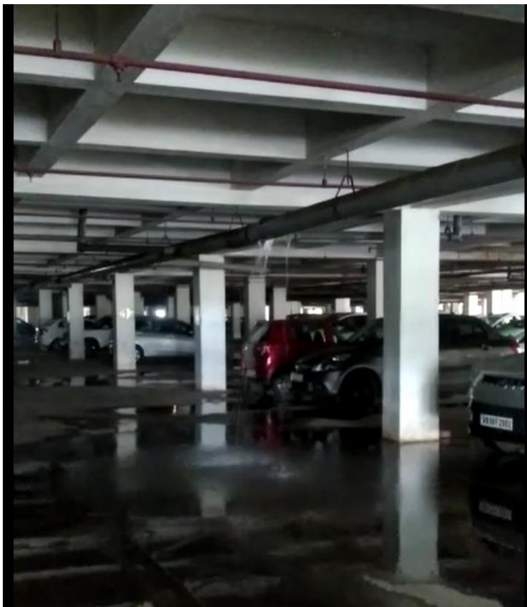
Water leakage from roof of covered parking during rainfall
