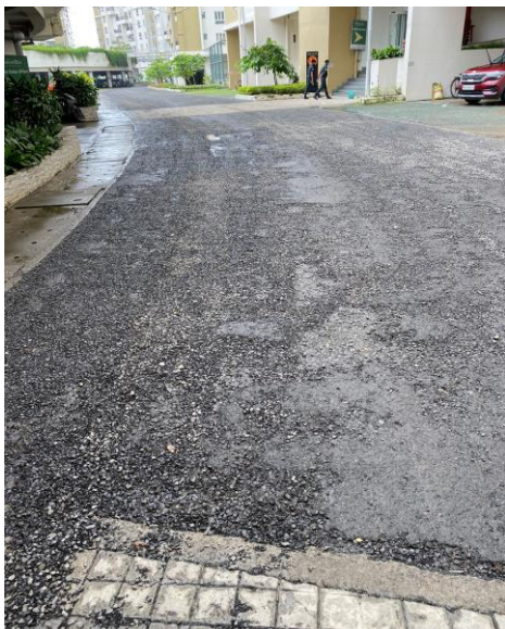
Poor Condition of Internal drive way
