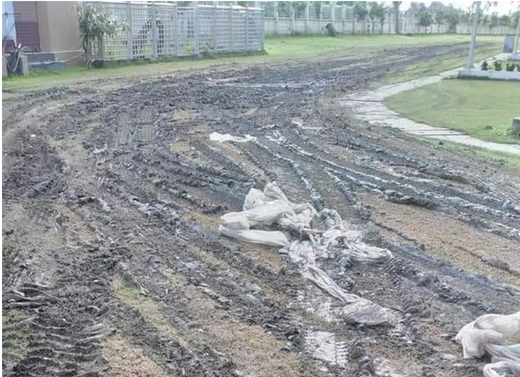
Poor Condition of Outer grass drive way
