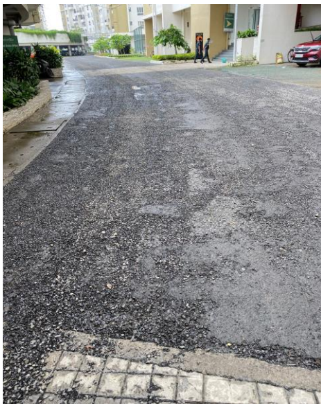
Poor Condition of Internal drive way
