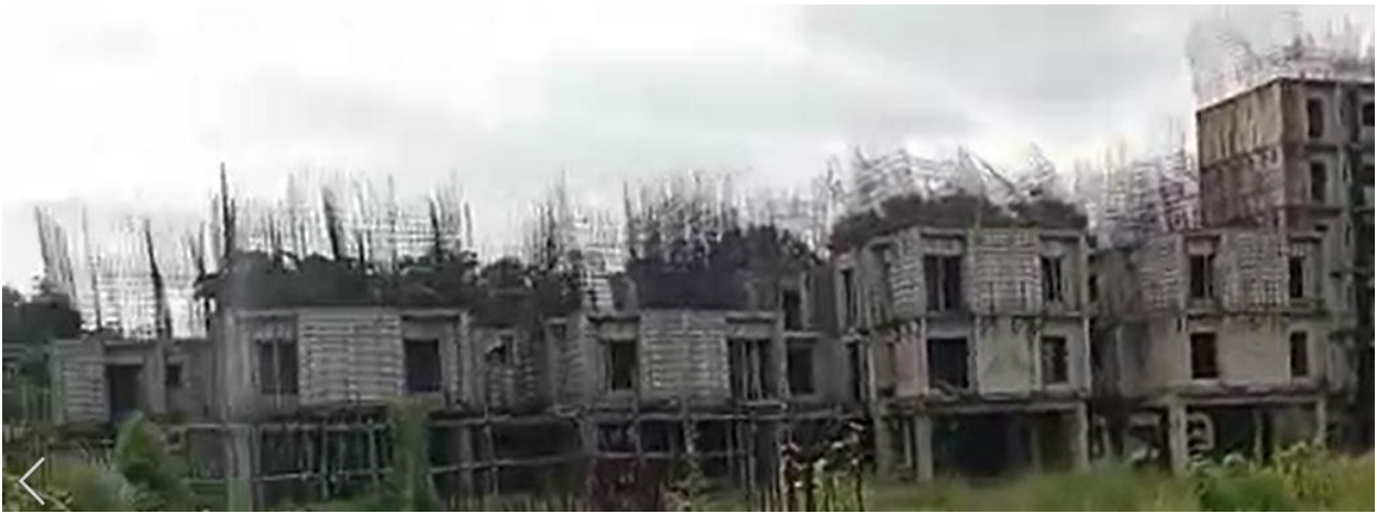
Plants & trees inside blocks & rusting TMT bars for 1 year
