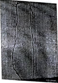
CRACKS ON WALLS.jpg 32K
