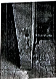
SEEPAGE AT MAIN ENTRANCE RT.SIDE.jpg 103K
